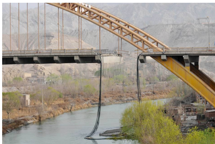
Figure 1.2 Failure of a bridge in service.
