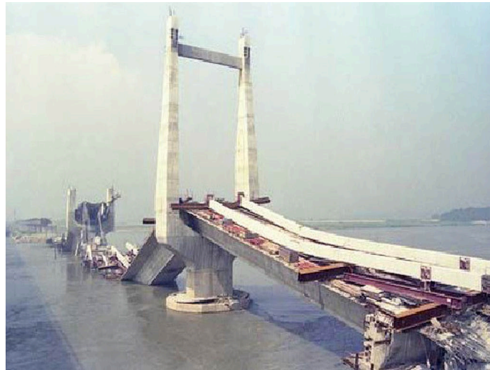
Figure 1.1 Failure of a bridge during construction.
